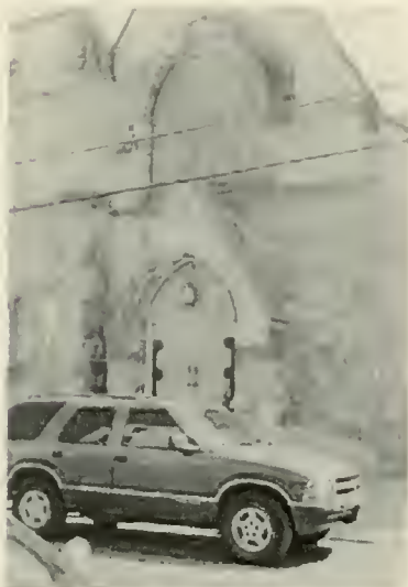
Figure 11 The main entry at the west side of the sanctuary shows surviving stucco above the belt course and exposed, deteriorating serpentine below.
